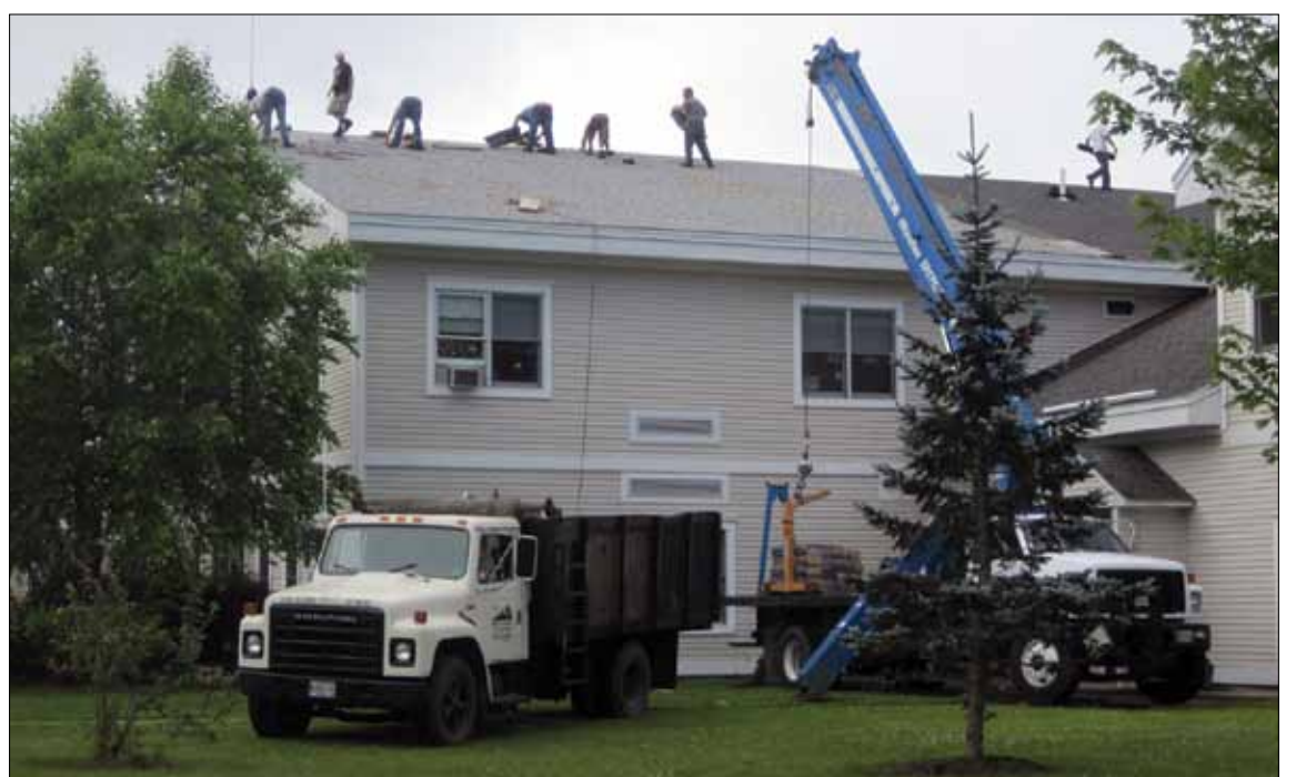
NEW ROOF AT SMITH SCHOOL —Workers from Roof Systems of Maine install a new roof on Leroy H. Smith School as part of a series of improvements funded by a QSAB bond issue that was approved by voters on June 11. The bond also funded security improvements at three RSU 22 schools. Story on page 4.
